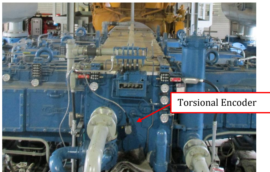
Figure 4: Torsional Encoder Installation on Auxiliary End of Compressor Frame
